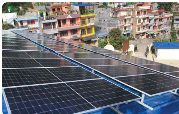
Gorkha Hospital in Gorkha Municipality-2 recently received a 64.8 kWp solar energy system, ensuring uninterrupted power supply.
