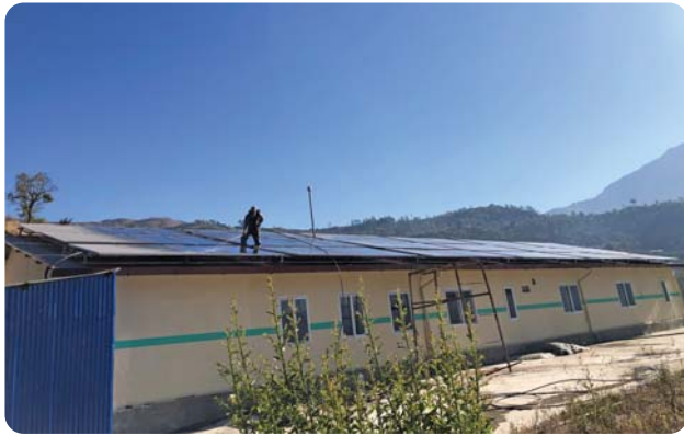
The remotely located Raskot Hospital in Kalikot now has electricity, courtesy of a newly installed 30 kWp Large Scale ISPS.
