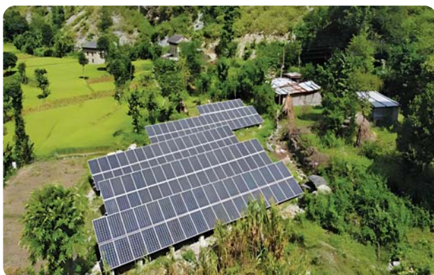
Solar panels with a capacity of 115.52 kWp installed in Sunkoshi, Ramechhap district as part of the large-scale RSDWP, serving 415 households.
