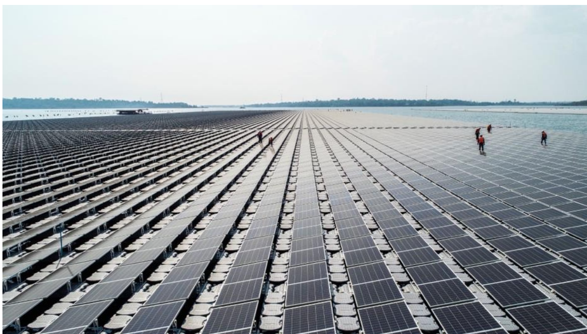
Figure 16: 45 MW floating solar at Sirindhorn Dam, Thailand 113
