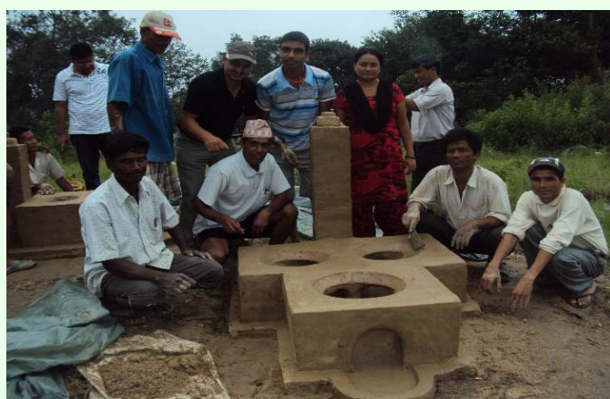
Figure:1 Participants of construction training on Institutional Improved Cooking Stove with the stove made by them during the training in Dhulikhel
