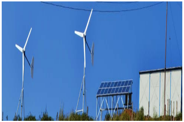
Wind Solar Hybrid System (Wind generators and Solar panels)
