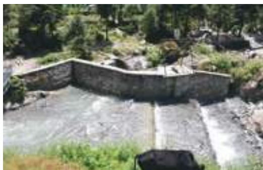
Figure 7: Headworks of Lower Bom Mini Hydro, Solukhumbu
