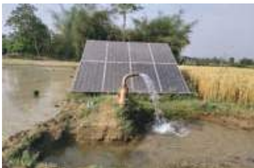
Figure 11: Solar Irrigation Pump
