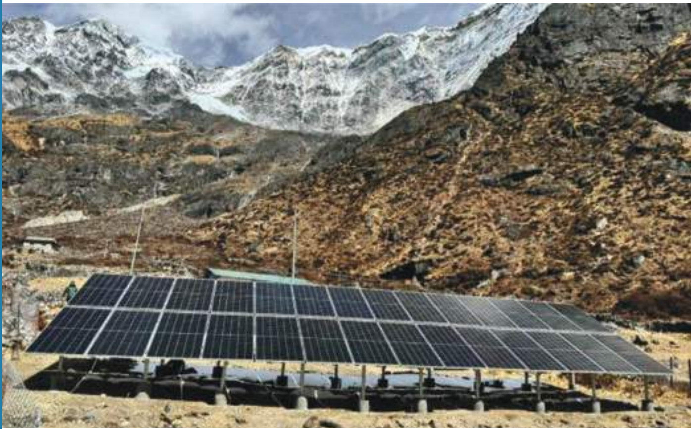
NA Village Solar Mini grid – 30kWp, Gaurishankhar Rural Municipality, Ward no-9, Dolakha District
