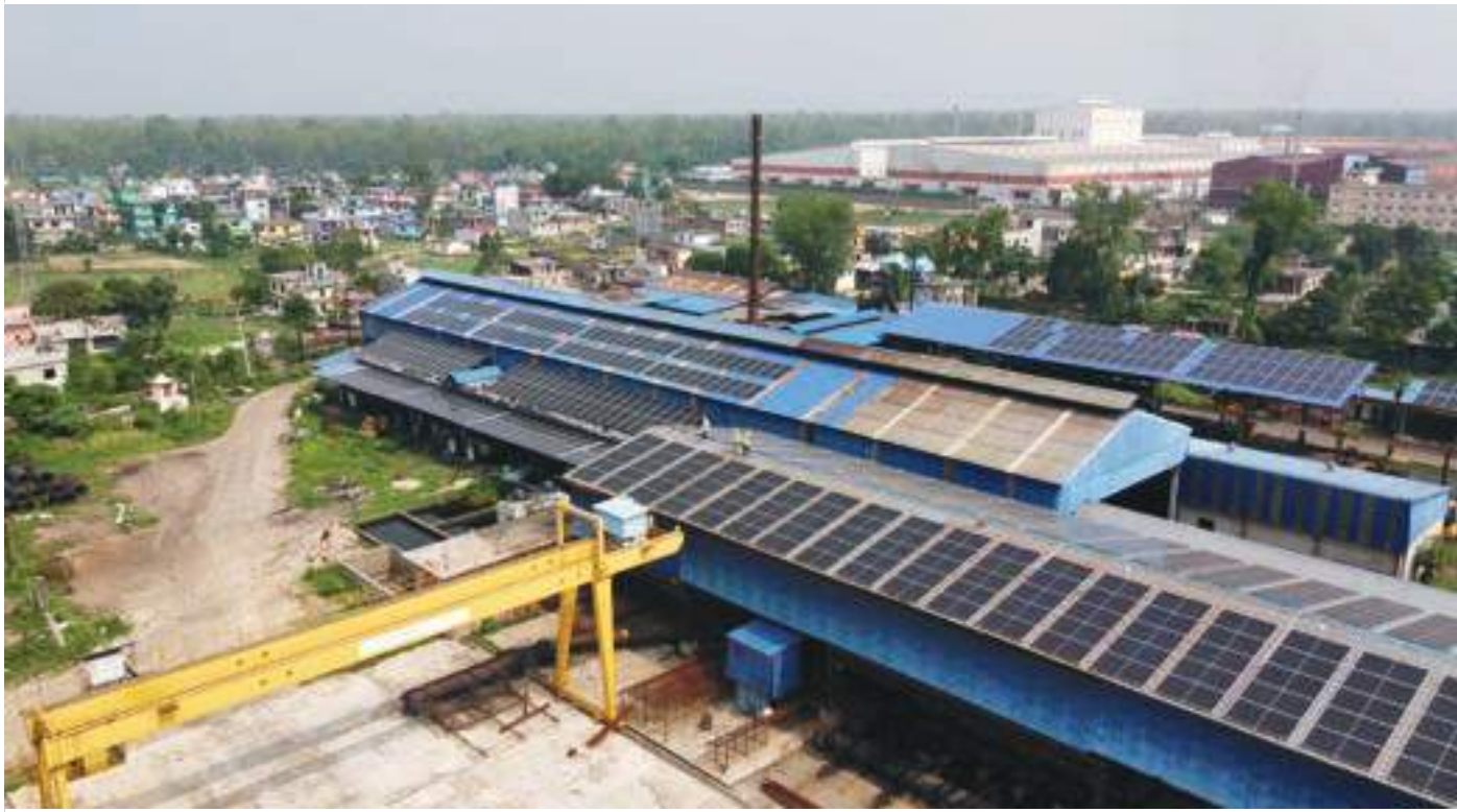
Solar Rooftop with capacity 633.6 kWp installed in Hama Iron and Steel Industries Simara, Bara with support from AEPC/KFW-DKTI Solar Project
