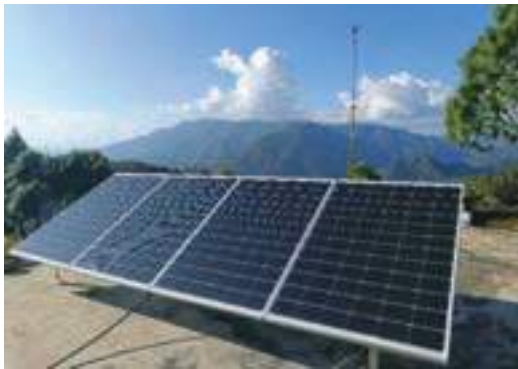
Figure 14: 1 kWp Institutional Solar PV System (ISPS)
