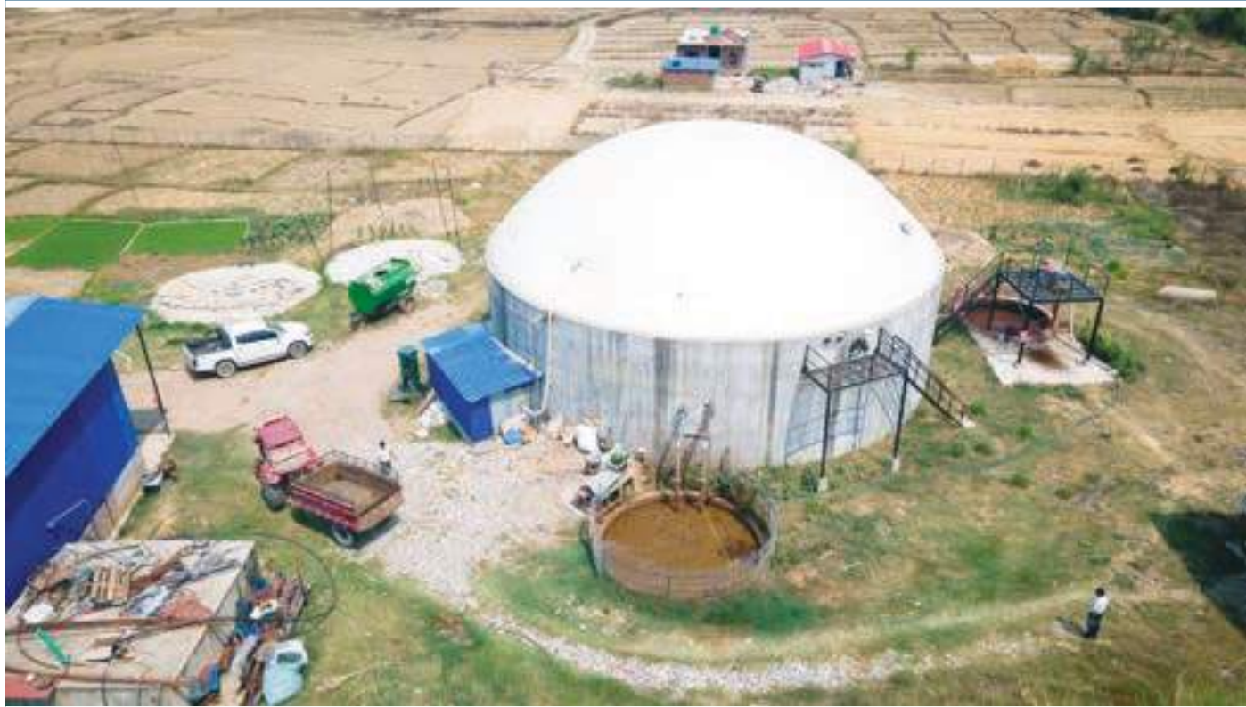
Municipal Waste to Energy Project (30 Tons Per Day-TPD), Birendranagar Municipality, Surkhet
