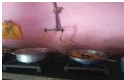
Figure 18: A biogas stove
