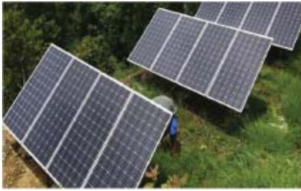
Figure 13: Solar panel mounted for solar pumping
