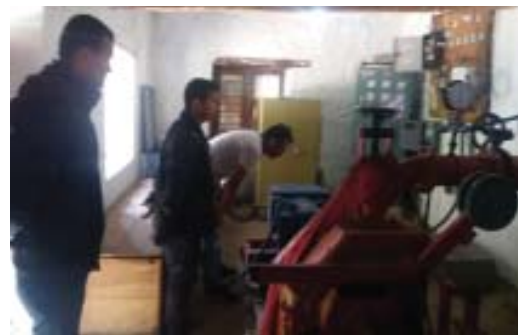
Figure 12: A typical MHP powerhouse
