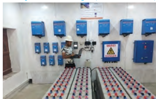
Figure 12: Battery and Control Room of 30kWp Malladehi Dandapur Solar Mini-grid (Purchaudi, Baitadi)
