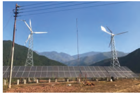
Figure 20: 15kWp Solar PV array and 20kWp Wind Turbine at Chisapani Village of Hariharpurgadi, Sindhuli
