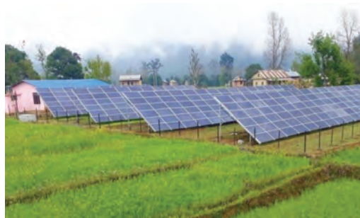
Figure 11: Solar PV Array and Powerhouse of 100kWp Gutu Solar Mini-grid (Chaukune, Surkhet)
