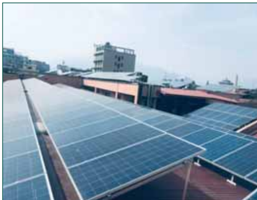
Figure 11: Grid connected solar
