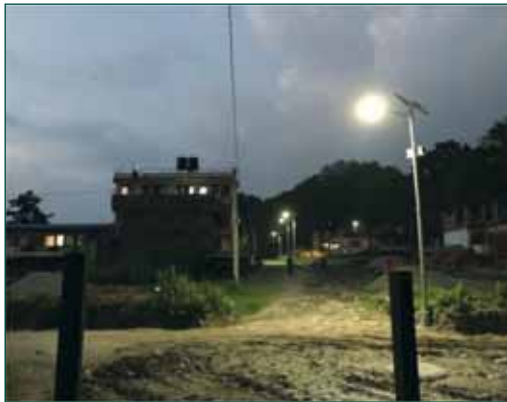
Figure 9: Solar Street Lighting supported by AEPC
