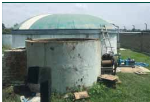
Figure 15: Large biogas plant
