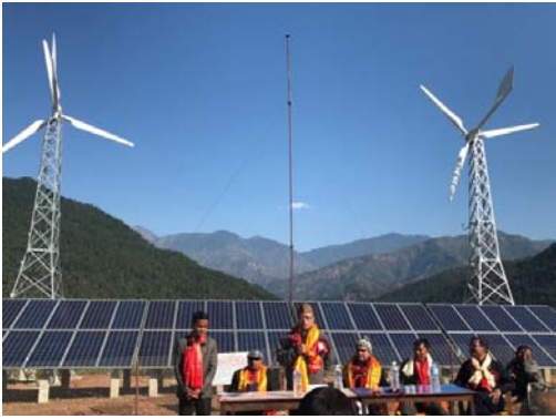
Figure 18: Solar Wind Mini Grid at Chisapani, Sindhuli
