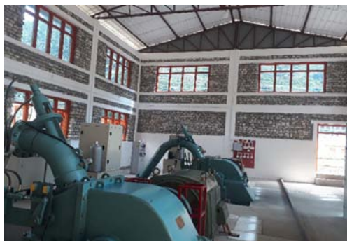
Figure 9: Inside view of 380 kW Tara Khola MHP
