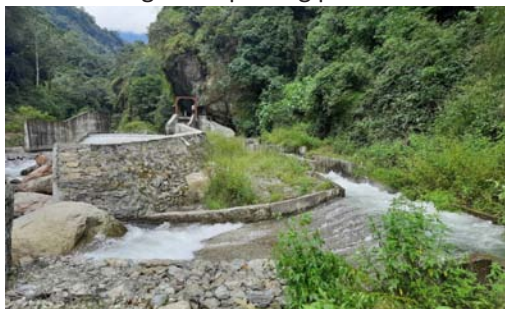
Figure 7: Headworks of 500 kW Middle PhawaKhola MHP, Taplejung
