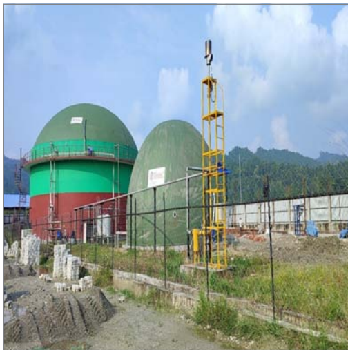
Figure 15: 40 TPD Biogas plant at Damak Municipality, Damak
