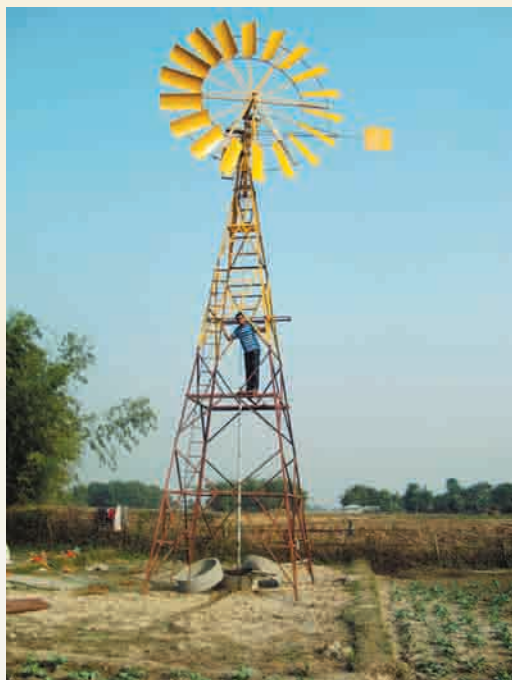
Wind pumping site at Bhaua VDC in Morang district.
