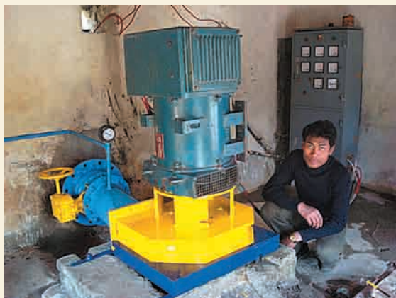
Micro Francis turbine at Handi Khola, Sindhupalchok.
