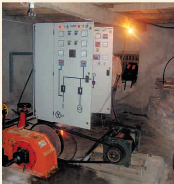
Grid Synchronisable PLC based control panel in Mini Grid Project, Baglung.
