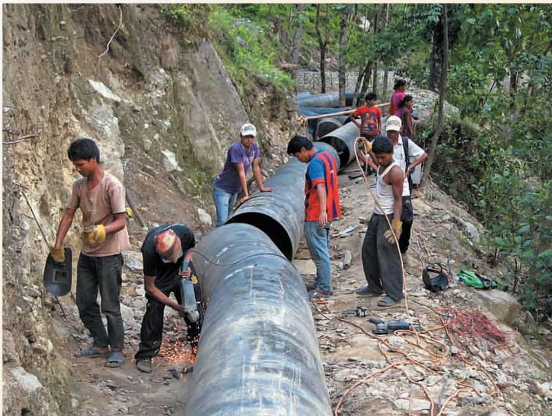
Construction Work at Haluwa Khola Mini Hydropower Plant, Namadi, Ramechap. Photo: KiND Project.
