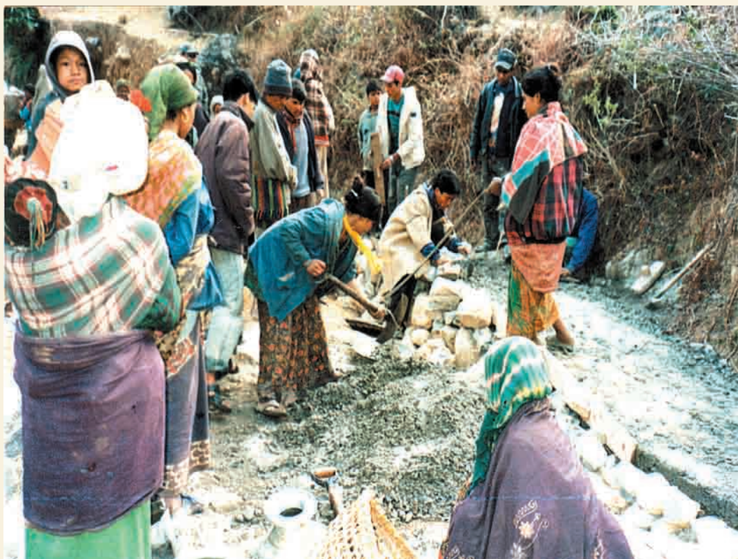
Members of the Users' Committee preparing construction material for of the 40kW Charibang Khola MHP, Baglung
