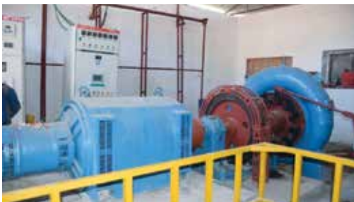
Figure 8: Inside view of 200 kW Giri Khola MHP
