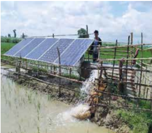
Figure 12: Solar Irrigation Pump
